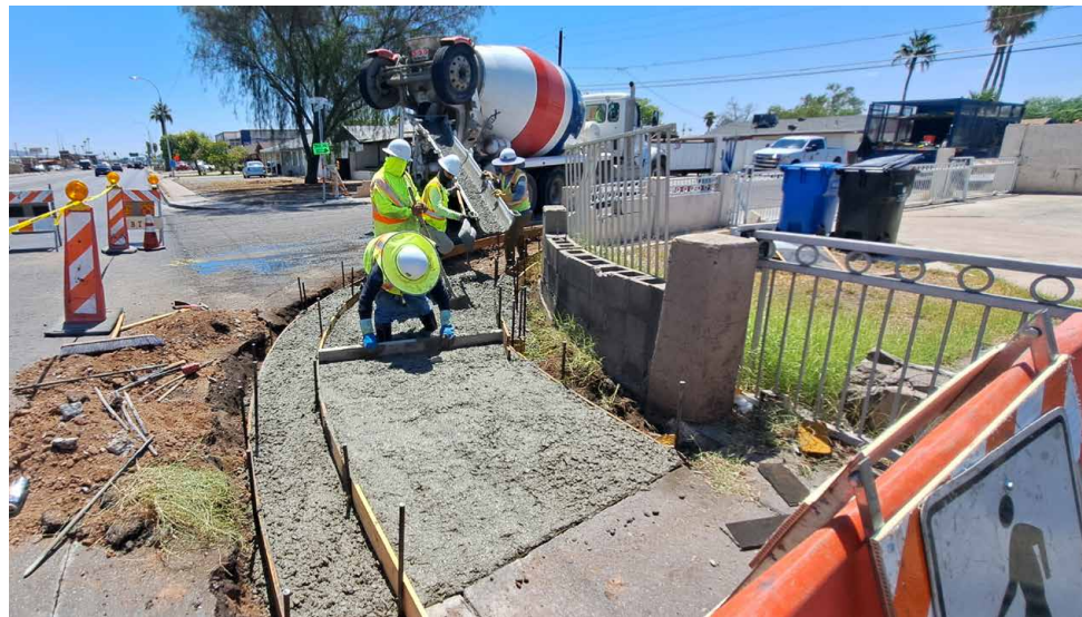
Construction crews are installing hundreds of ADA curb ramps throughout the city, eliminating barriers to mobility for people with disabilities.
